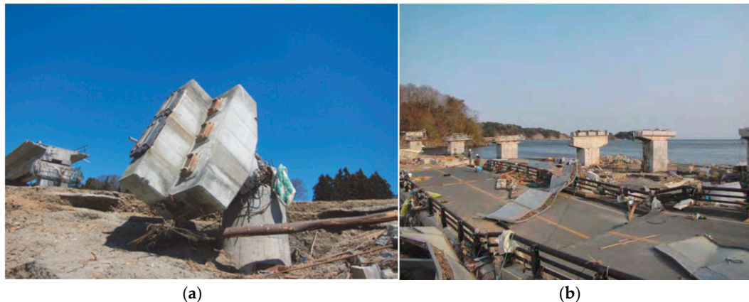
Figure 1. (a) Damaged piers of the JR Rail Viaduct at the Tsuya River (photo: S. Dashti); (b) Damages to the deck and piers of Utatsu Bridge (Photo: Kenji Kosa).
