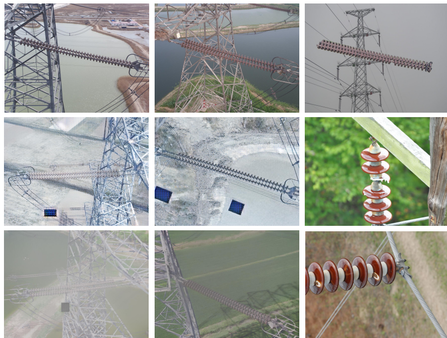
Figure 5. The multi-domain insulator dataset (MD-Insulator) contains 12,605 insulator images with three common insulator defects: self-explosion, flashover damage, and broken insulator.
