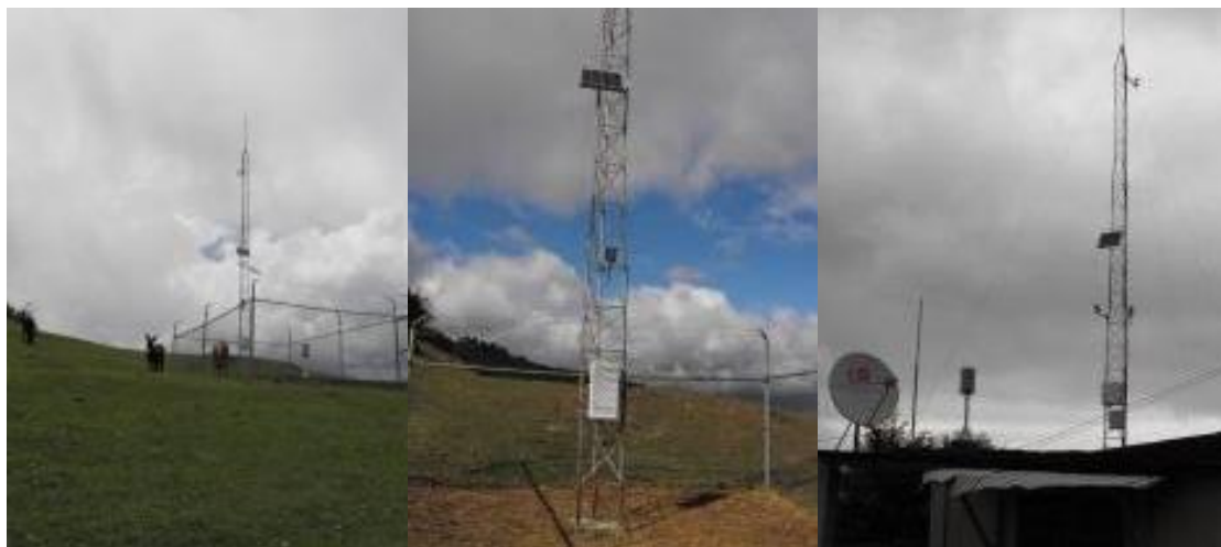
Figure 19. Photographs of the installed RTUs.
