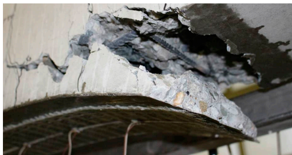
Figure 13. Failure of the RC beam strengthened with textile sensor.
