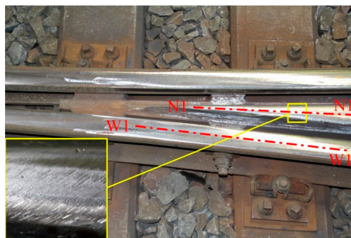
Figure 11. Repaired crossing profile with a magnified image of grinding marks. The degraded crossing was repaired through a grinding-welding-grinding process: first, rail surface damages were removed via grinding; second, hollow regions were filled by welding material; last, the rails were ground again to shape the profile.
