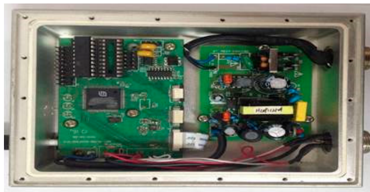
Figure 9. Internal structure of data station.
