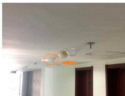
Figure 6. A signal transmitter in the corridor.
