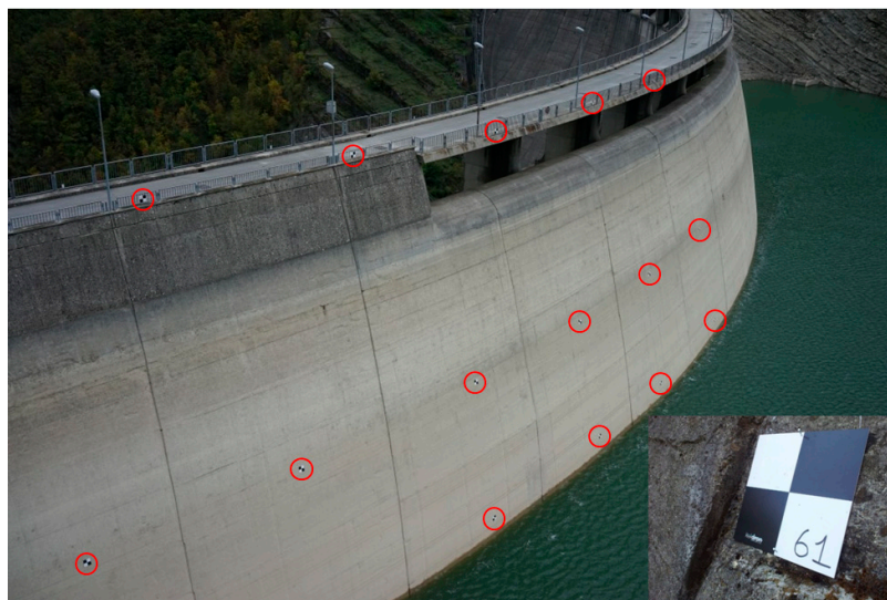
Figure 3. Upstream face of the Ridracoli dam. The red circles indicate marker positions. The small panel shows a marker applied on the structure.
