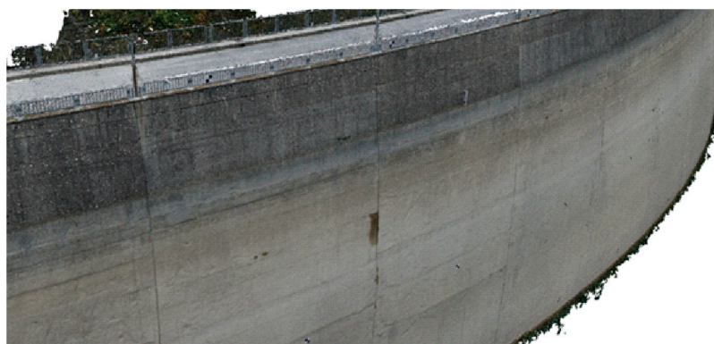
Figure 7. UAV dense 3D point cloud of a portion of the upstream face of the Ridracoli dam.
