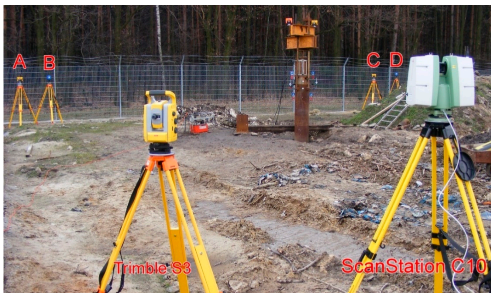
Figure 7. The geodetic instruments (total station Trimble S3 and laser scanner Leica ScanStation C10) with some reference points and self-balanced testing appliance.
