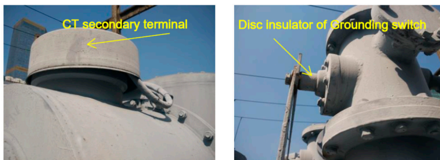
Figure 11. Appearance of CT secondary terminal and disc insulator of grounding switchgear.
