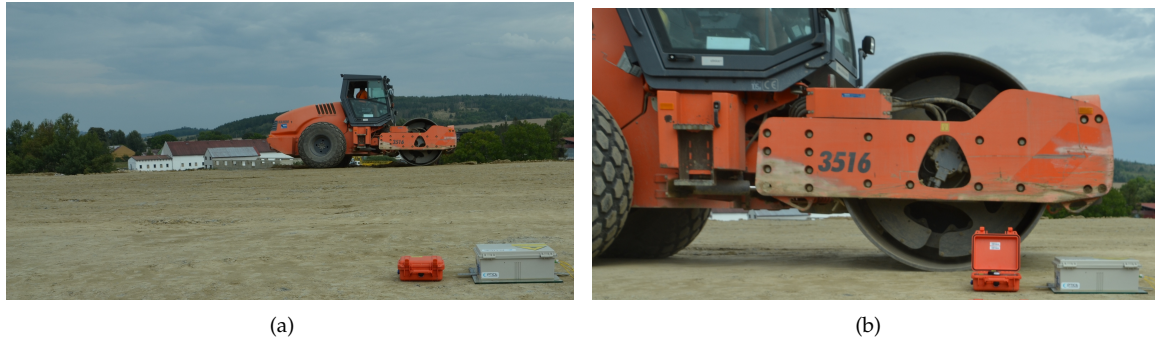
Figure 4. Photo documentation taken during the comparative measurement: (a) maximum distance of the vibrating roller from the measuring equipment: 13.5 m; (b) the minimum distance of the vibrating roller to the measuring equipment: 1.4 m.
