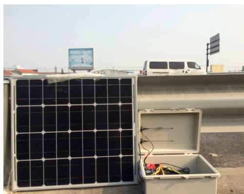
Figure 16. The gateway installation.
