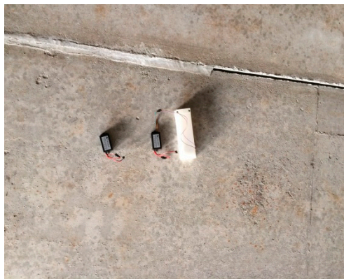
Figure 15. The sensor installation.
