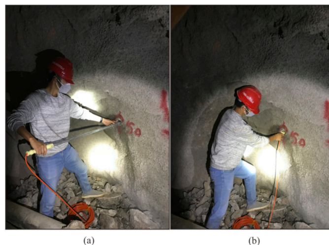
Figure 10. The semi-automatic coupling geophone installation in the tunnel: (a) before, (b) after installation.
