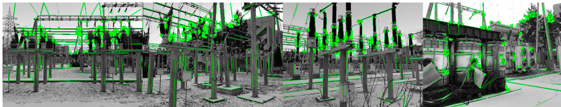
Figure 13. Feature extractions of the VIO front-end in the substation scene.
