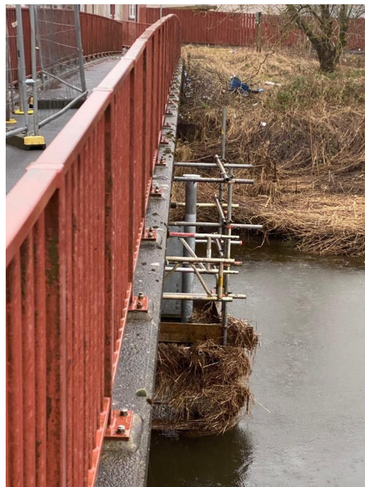
Figure 24. Hay and debris on the Probe 2.
