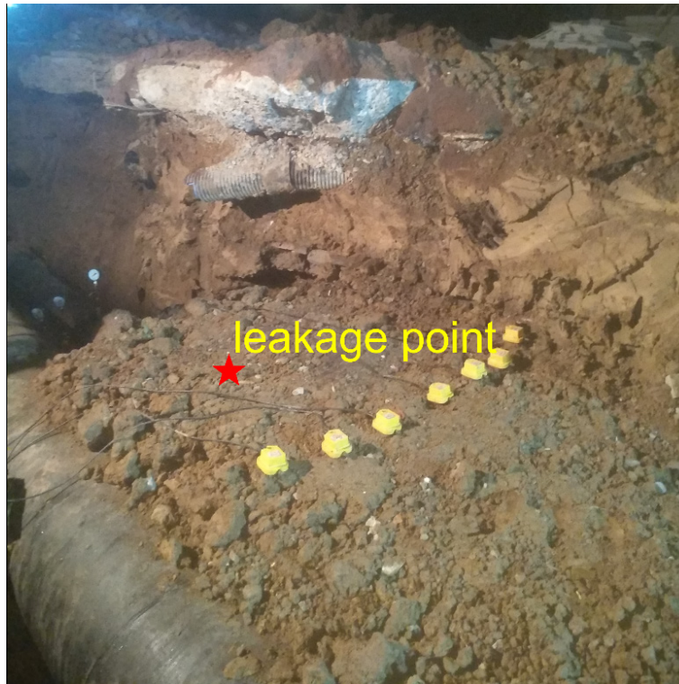
Figure 7. Ground surface vibration measurement using the sensor array at the distance of 0.5 m from the leak.
