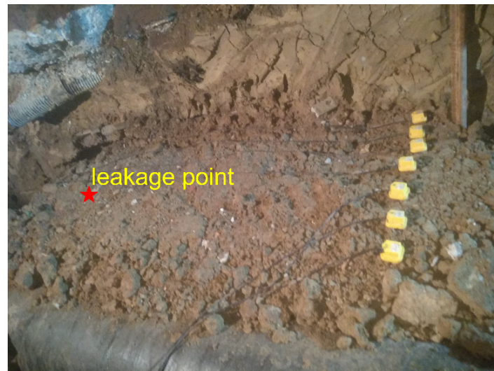
Figure 5. Ground surface vibration measurement using the sensor array at the distance of 1.5 m from the leak.
