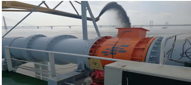
Figure 7. The \gamma -ray sensor in the pipeline.
