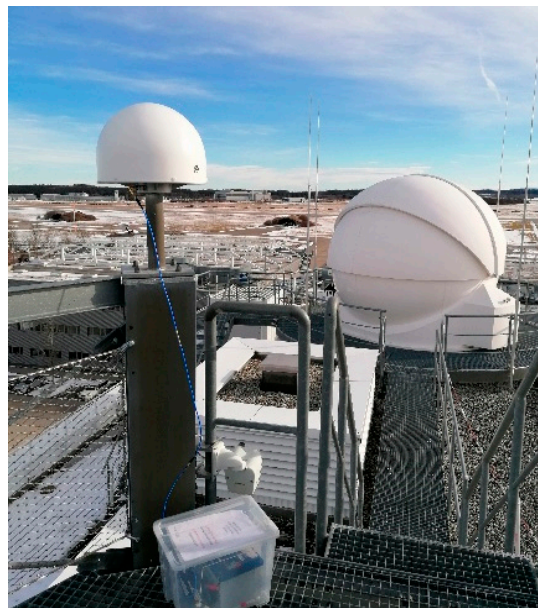
Figure 11. Example of reference antenna mounted in a more challenging environment, in this case, the rooftop of DLR's Institute of Communications and Navigation.
