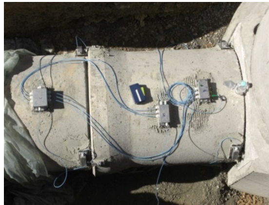
Figure 12. Example of a quasi-distributed FBG sensor network that was developed for the SHM of sewerage tunnels. Reprinted with permission from Ref. [68]. Copyright 2016 Procedia Technology.
