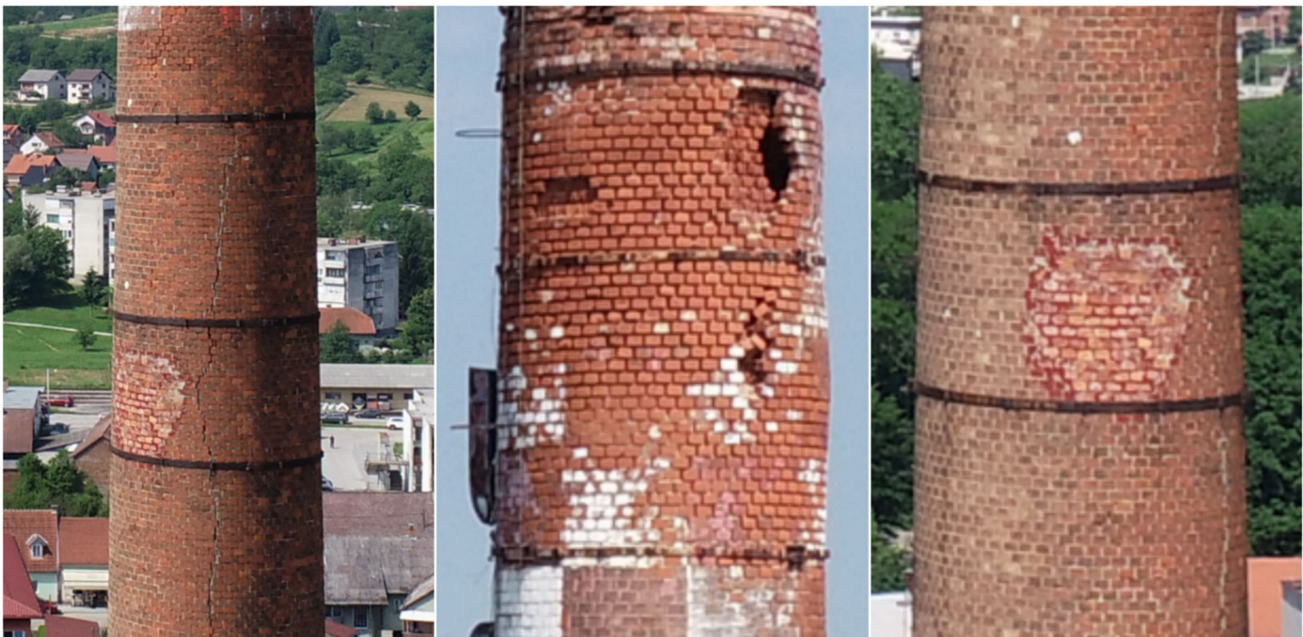
Figure 2. Current condition and structural damage of the studied industrial masonry chimney of the former Duga Resa Cotton Industry in Duga Resa, Croatia.
