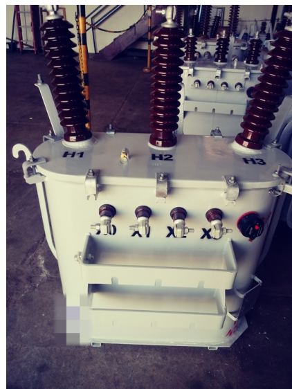
Figure 7. Picture of the transformer considered in the experiment.
