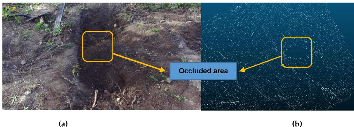
Figure 3. Example of an occluded region on the excavation site: (a) Indication of a pile that blocks the sensor vision causing occlusion; (b) Initial exteroceptive map using LiDAR sensory data (point cloud) for the same site that includes the identical occlusion region.
