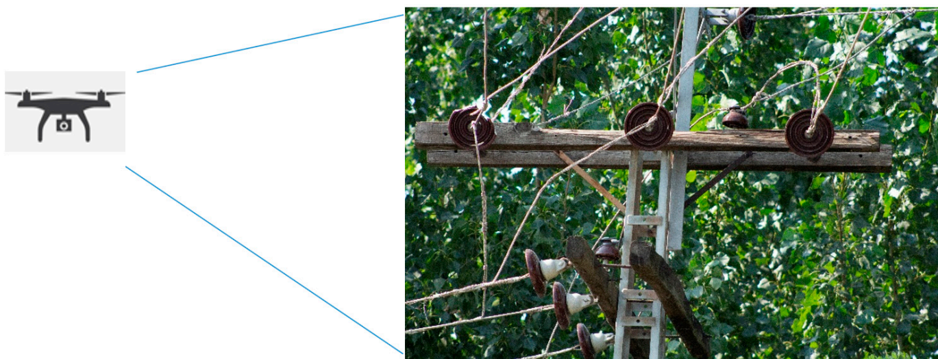
Figure 2. Illustration of overhead power distribution line from drone camera.
