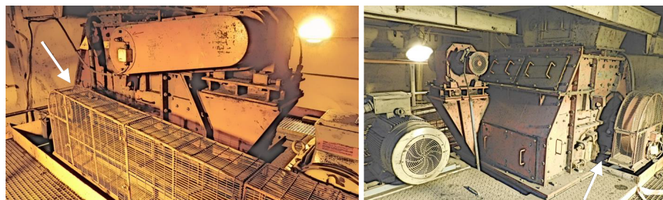
Figure 4. Photography of both sides of the monitored crusher—the approximate location of the sensors is indicated by arrows.
