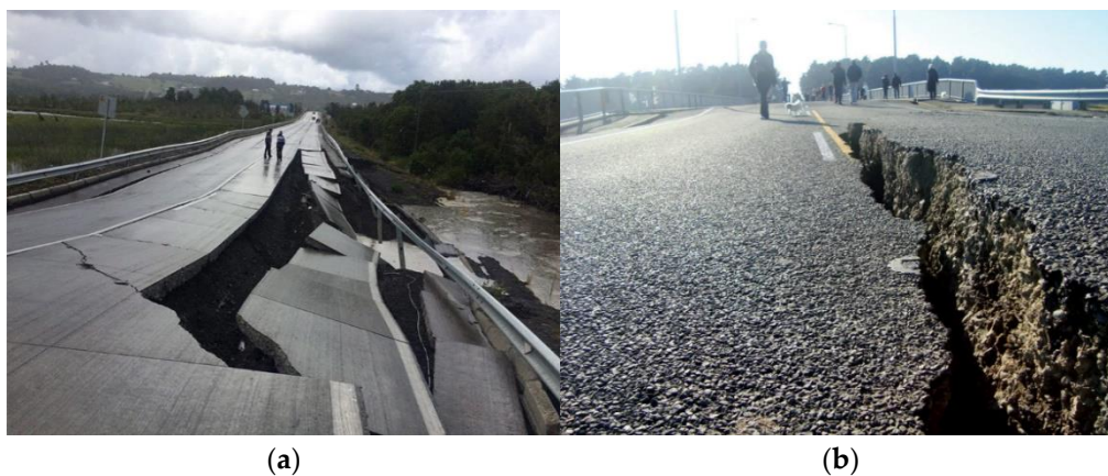
Figure 4. (a) Depicts a severely damaged bridge after an earthquake in New Zealand. (b) Depicts a mildly damaged bridge after an earthquake in Chile.
