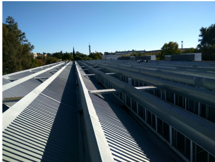
Figure 2. Photograph of the roof of the Leonardo da Vinci building of the Rabanales University Campus of the University of Córdoba (Spain).
