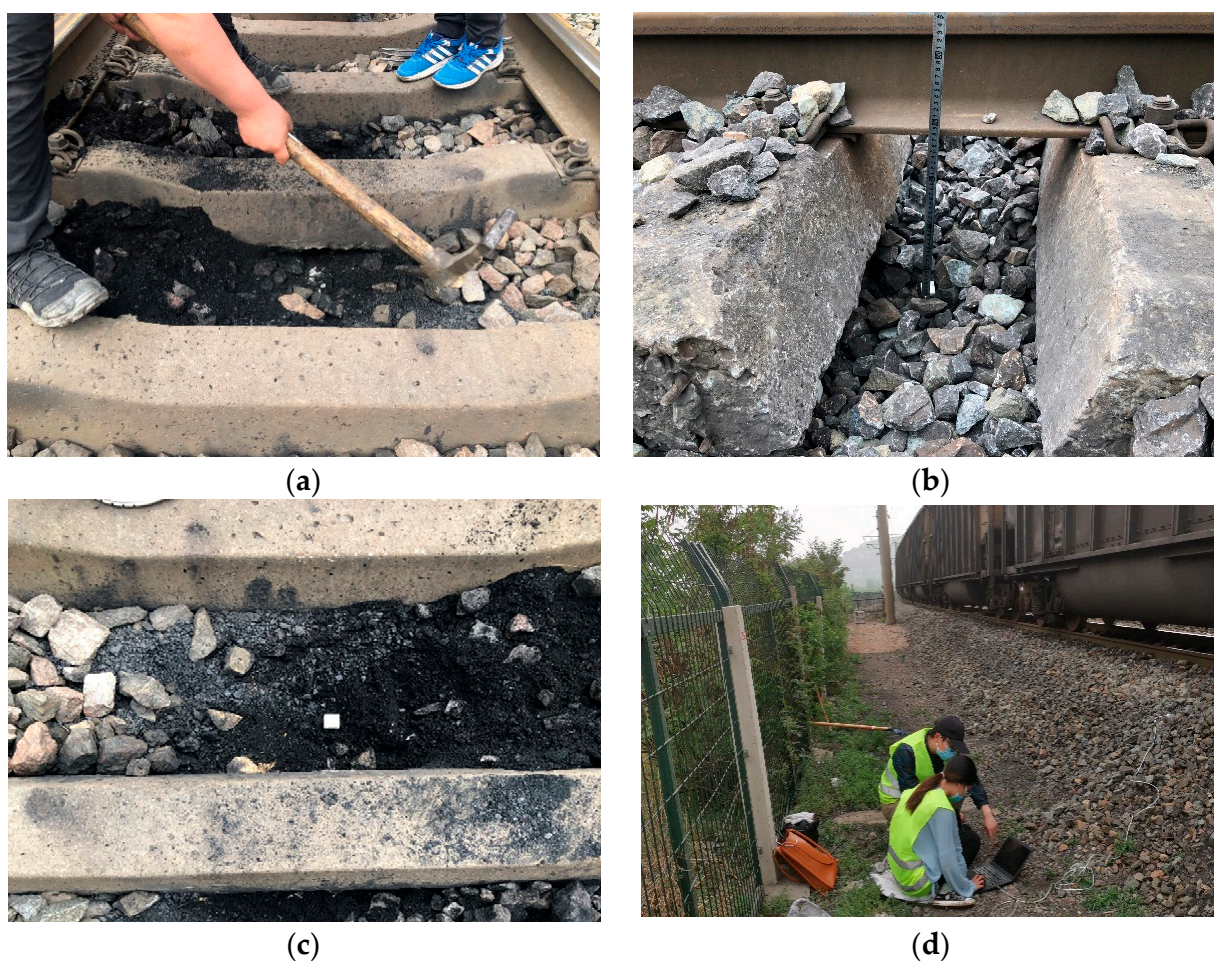
Figure 7. Field Installation sequences of the SR sensors: (a) Instrumentation excavation; (b) Sensor placement; (c) Ballast backfill; (d) Data acquisition.
