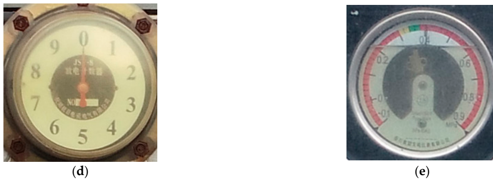
Figure 3. Five kinds of meters. (a) bj, which refers to oil level, (b) bjA, which refers to Sulfur Hexafluoride Density Relay, (c) bjB, which refers to Discharge Counter With Current Meter For Arrester, (d) bjH, which refers to Discharge Counter and (e) bjL, which also is Sulfur Hexafluoride Density Relay.
