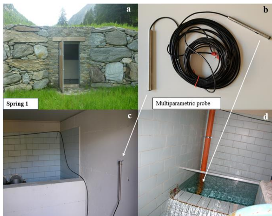
Figure 3. Mascognaz 1 spring's structure and set up: (a) External view of the spring water intake structure; (b) Multiparametric probe geometry; (c) Installation of probe data logger; (d) Installation of recording probe.
