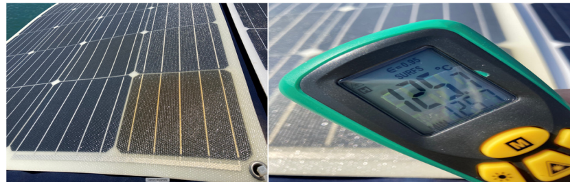
Figure 19. Brownish effect and temperature on a cell after a day of its installation.
