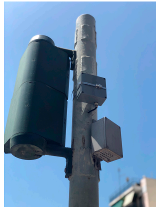
Figure 8. Specially mounted external device on a real traffic light located at the junction of Doiranis and Athinas in Kallithea.
