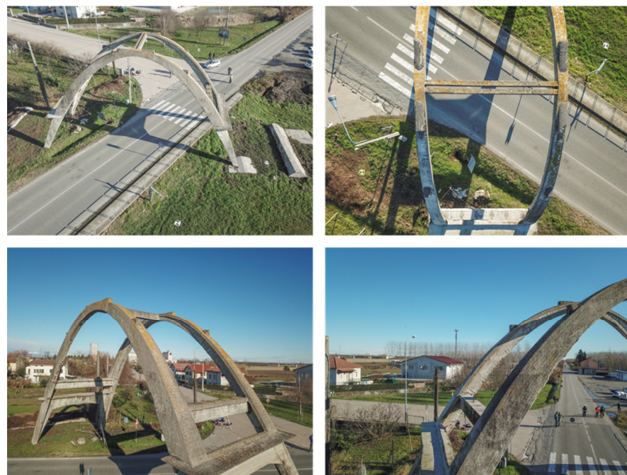
Figure 4. Digital images acquired from an aerial perspective using the micro UAV system, which enabled the acquisition of the extrados and the higher surfaces of the concrete arch.
