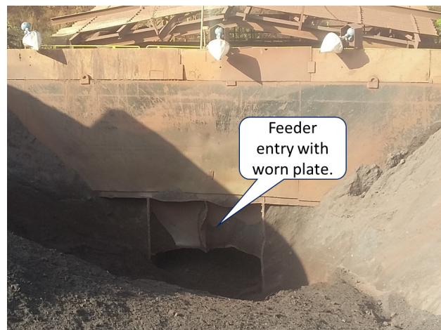
Figure 6. Feeder inlet with worn plate from the feeder–conveyor system under study.
