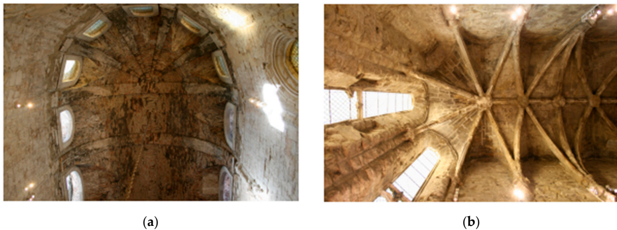
Figure 6. Details of the chapels: (a) masonry barrel vault covering the main apse; (b) example of the limestone ribbed vaults covering the secondary chapels.
