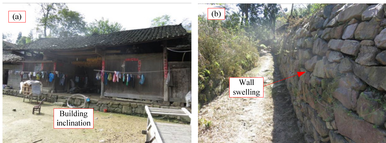
Figure 6. Phenomenon in front of landslide, (a) Building inclination, (b) Wall swelling.
