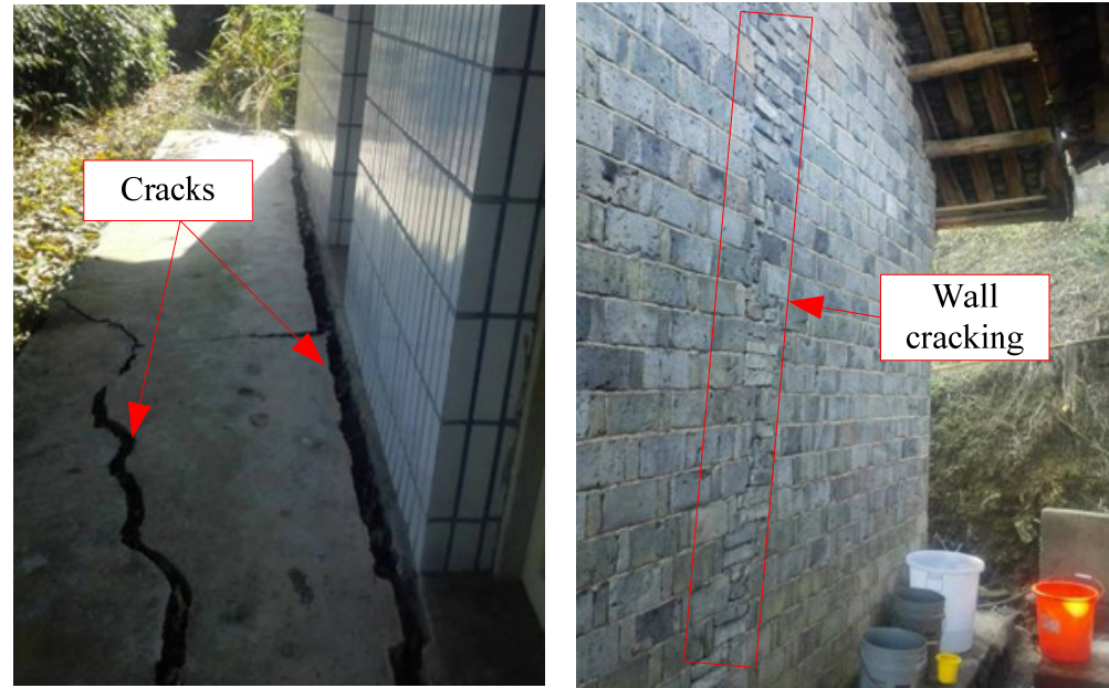
Figure 5. Cracks on wall and ground.
