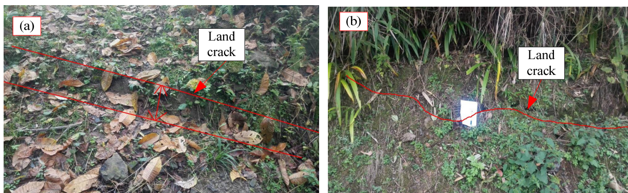
Figure 3. Cracks induced by landslide: (a) Cracks in rear edge of landslide, (b) Cracks in front edge of landslide.
