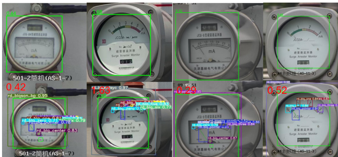
Figure 7. YOLOv5-MRL recognition effect. The first and third columns of the above diagram show the JCQ-8 lightning rod monitor and the second and fourth columns show the JCQ3A lightning rod detector. The first row is the original picture and the second row is the schematic of the test result. Where rd_blq_zero means scale 0, rd_blq_one means scale 1, rd_blq_onefive means scale 1.5, rd_blq_two means scale 2, rd_blq_twopfive means scale 2.5, rd_blq_three means scale 3, rd_blq_four indicates scale 4; rd_blq_s, rd_blq_five means scale 5, rd_blq_six means scale 6.
