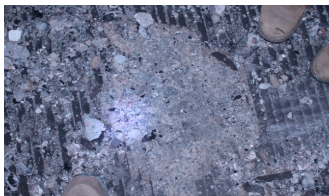
Figure 5. Ablation condition of surface concrete.
