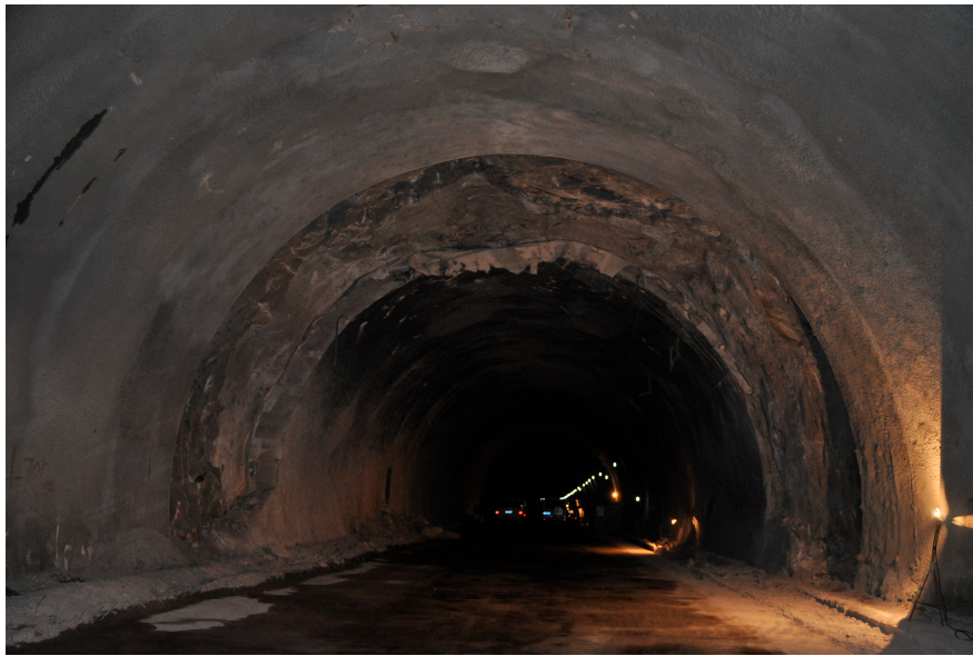
Figure 2. Lining of New Qidaoliang Tunnel after the fire.
