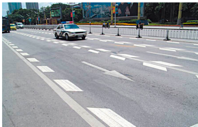
Figure 1. Longitudinal speed reduction markings (LSRMs) in China.
