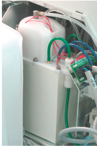
Figure 1. The Water Hygienization Equipment (W.H.E.) device inside a dental unit, at the inlet of the municipal water.
