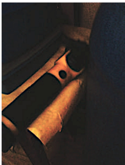
Figure 6. The interior of Joan’s ‘hot-press’, displaying the central heating timer and immersion heater on the left, and torch on the right. Permission granted by Dr. L Shore.
