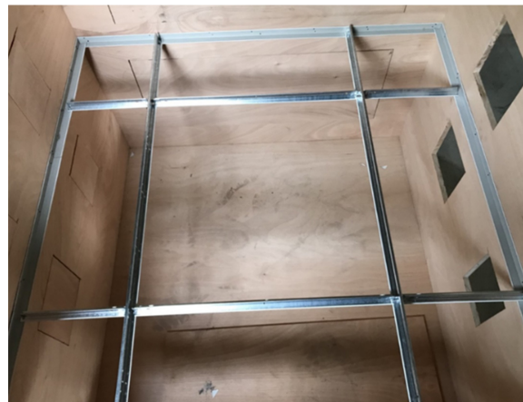
Figure 3. Installation of open-frame ceiling main frame and subframe in the test chamber.
