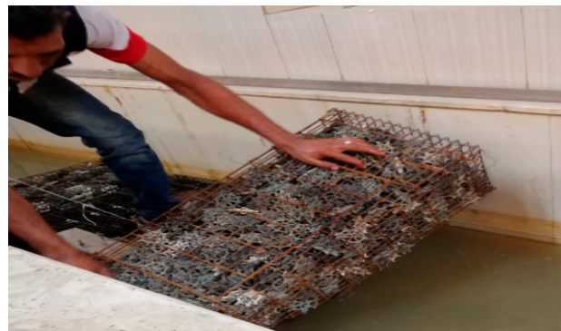
Figure 3. The galvanized steel mesh cages supporting the media installed in the channel.
