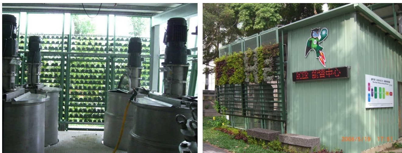
Figure 7. Experimental bio-hydrogen production plant (Left, Interior; Right, Exterior).
