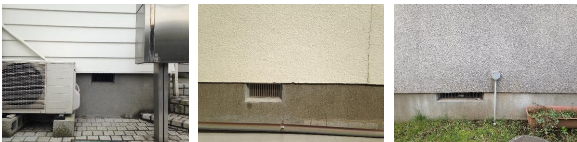
Figure 2. Underfloor openings for the natural ventilation in Tokyo, Japan.
