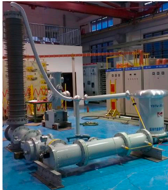
Figure 1. Photograph of the GIS tank.
