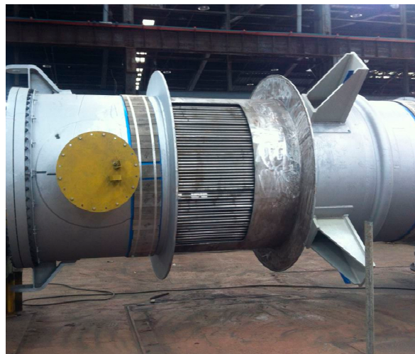
Figure 6. The side of the heat exchanger was open to install additional support grids to inlet vapor belt.
