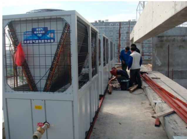
Figure 4. Air source heat pumps.
