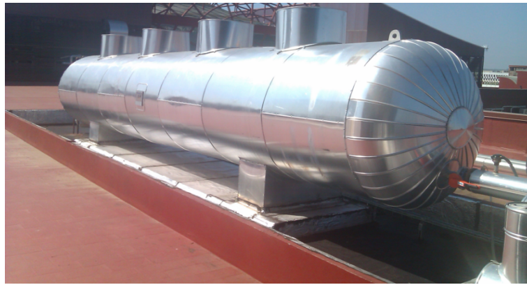
Figure 3. Phase change material (PCM) storage tank.
