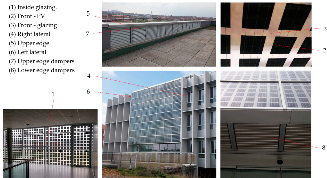
Figure 1. Different views of the ventilated façade with photovoltaics (PV) modules and zones studied in the model.
