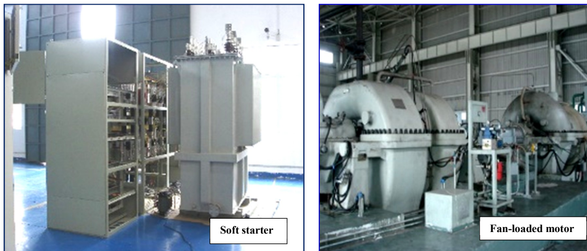
Figure 19. Soft starter and load of 10 kV/19,000 kW motor (picture).
